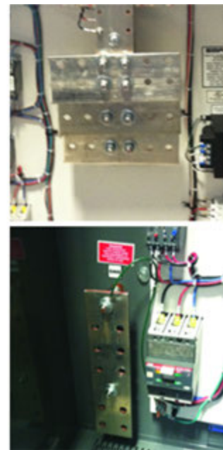
Main Bus (top) and Ground Bus
