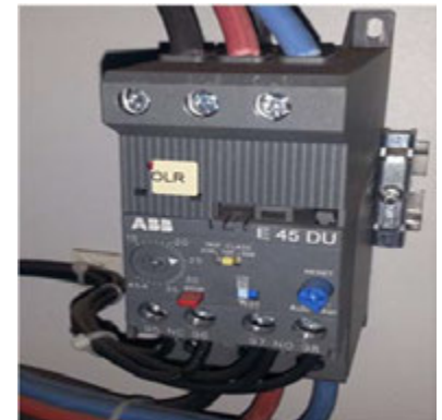
Overload Relay (OLR)
