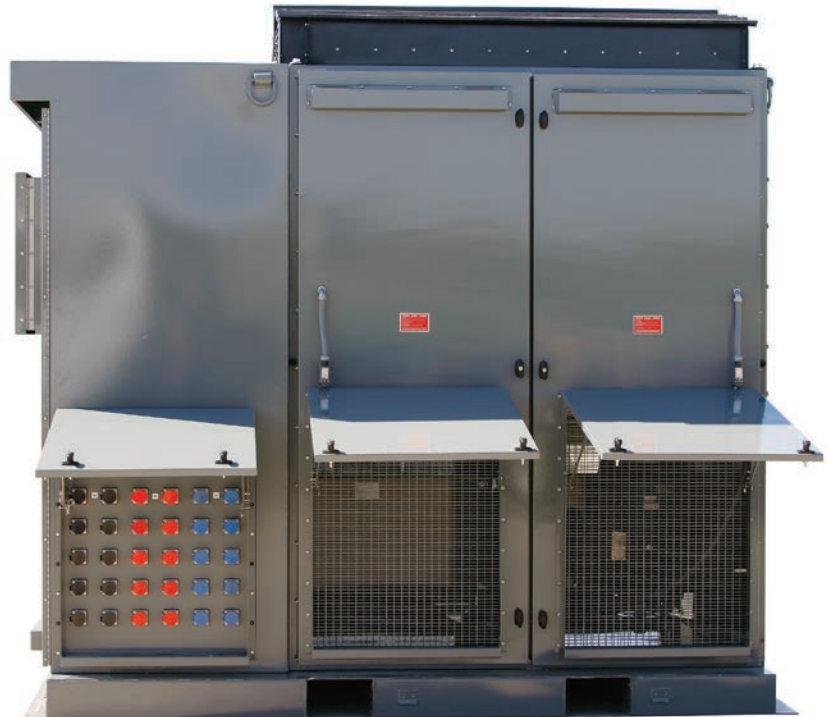
Right Side View with Cam-Type Connectors and Fan Intake Doors Open
