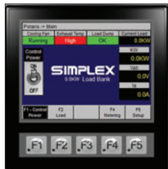
Figure 38 Exhaust Temp High
