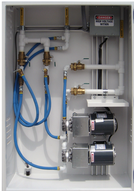
SPS-25-SD Mechanical Compartment
