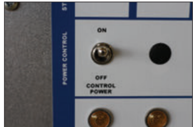
Figure 9 Control power switch
